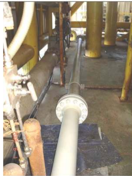
Transition of the final section to the middle one with the work done
