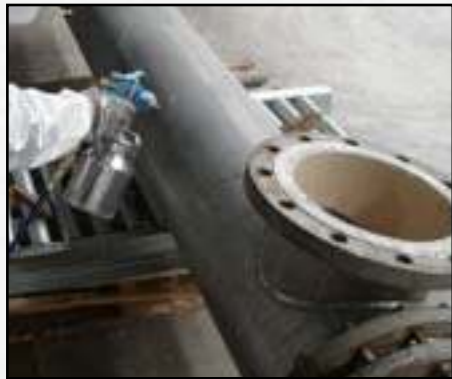
Insulation & Corrosion Control Guadalajara, Mexico
