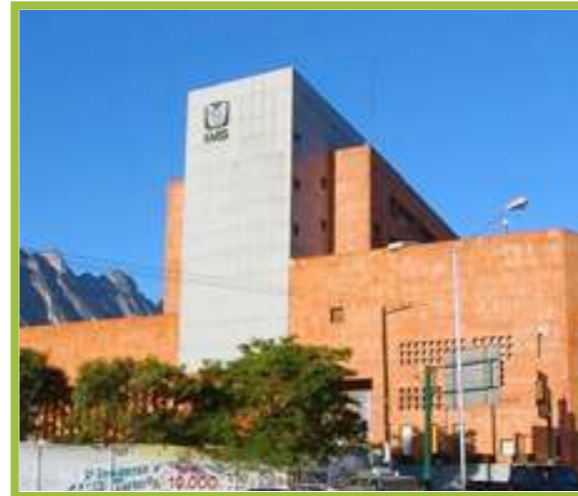
Data Center Roof Insulation Mexican Govt. - IMSS Monterrey, Mexico
