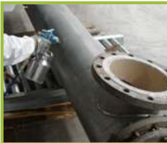
Insulation & Corrosion Control Grupo Modelo (Corona Beer) Guadalajara, Mexico
