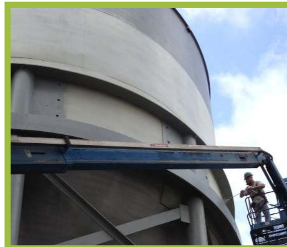
Tank Insulation Weyerhaeuser Pulp/Paper Savannah, Georgia, USA
