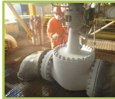
Steam System Insulation Pemex - Offshore Mexico
